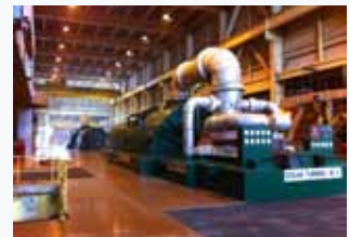
The Auraiya Gas Turbine Combined Cycle Power Station (India)
