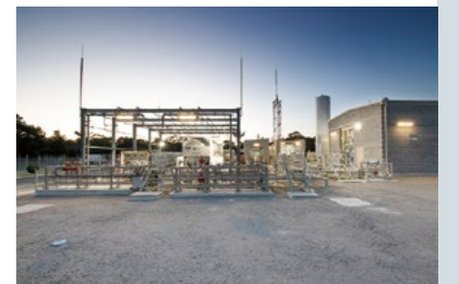
Hydrogen liquefaction and loading facilities in Australia (photo courtesy of HEA)
