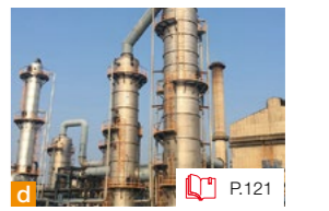
Image d: Facility that uses CO 2 capture technologies supplied by Carbon Clean Ltd. P.121
