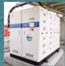
Hydrogen supply chain project (water electrolysis facility in Tomiya, Miyagi Prefecture)
